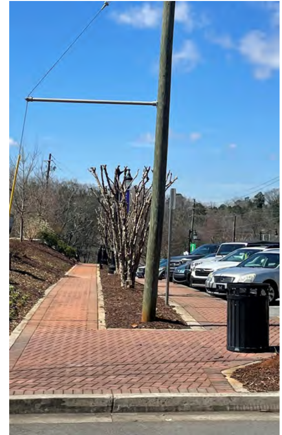
Missing Ramp at the corner of North Street and Academy Street
