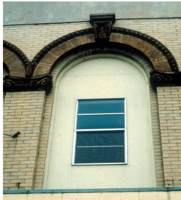
New or replacement windows should fit the original window frame. This window has been filled inappropriately with a stock replacement window.
