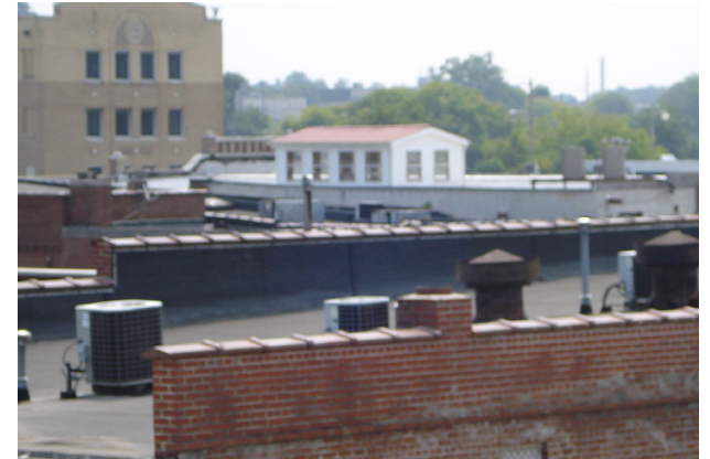
Mechanical units, such as air conditioning units or ventilators, should be located on roof tops.
