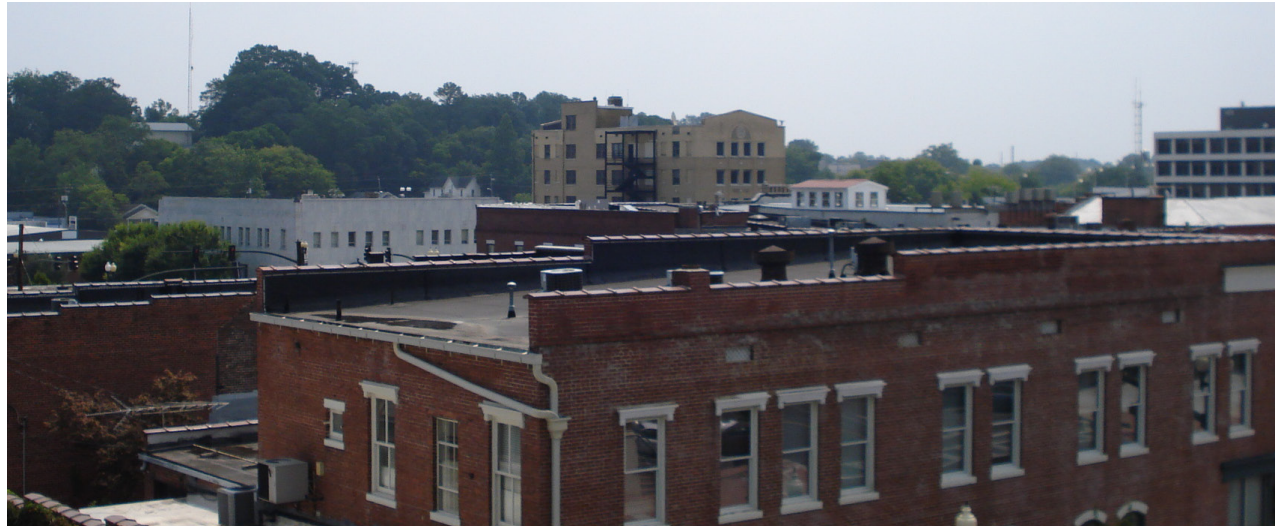
A well-maintained roof that slopes to the rear of the building helps divert water off and away from the building. Utilities are typically placed on the roof, but they should be placed so that they do not impact the function of the roof and should not be visible from the street.
