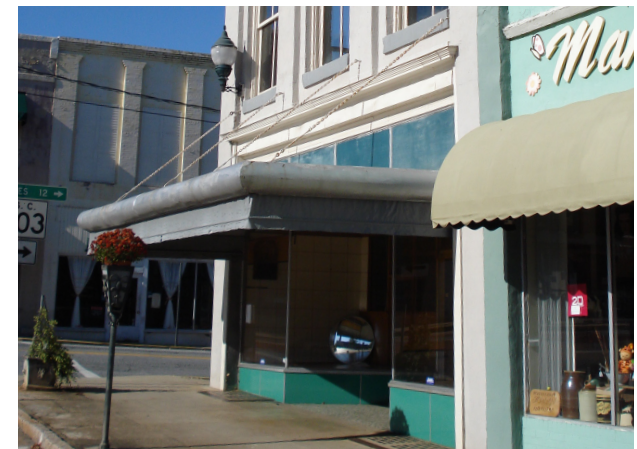
Canopies should be placed so that they do not obscure architectural features, such as transom windows or sign bands.
