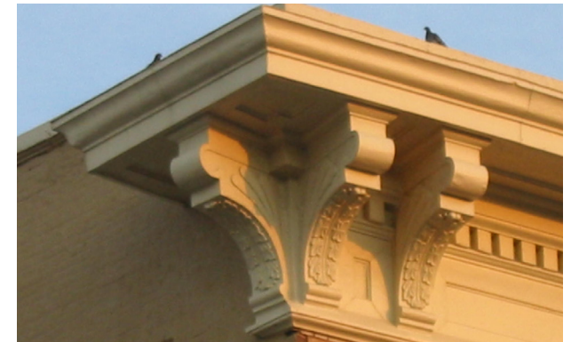
Traditional cornices commonly include decorative detailing with wood, masonry and/or stone treatments.
