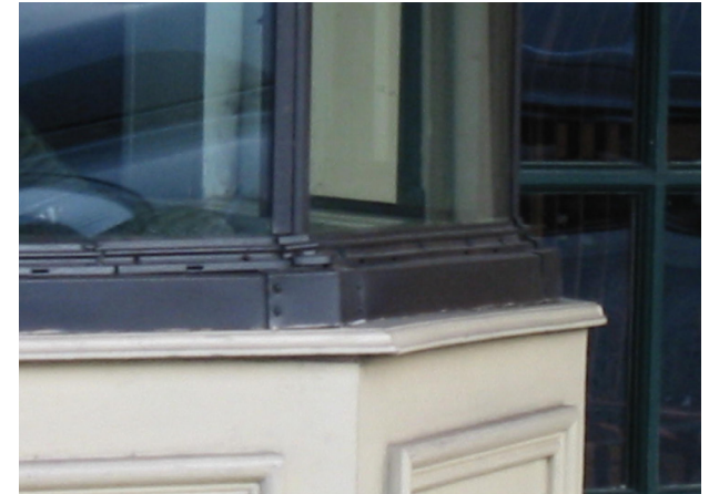
Display windows are often set to bulkheads using metal joints and material finishes.
