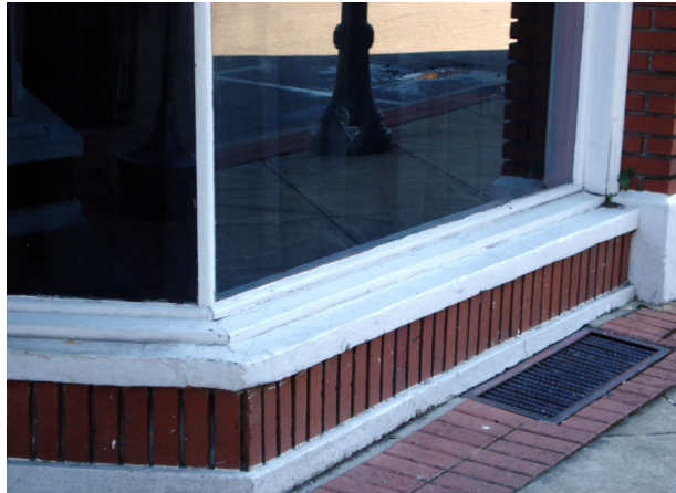
Bulkheads use a variety of construction methods and materials including wood and brick.
